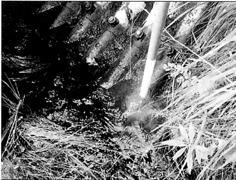
Photo 11 – Far Right End Perforation Holes in Floor
