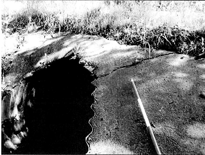
Photo 10 – Left Headwall Cracking. Typical
